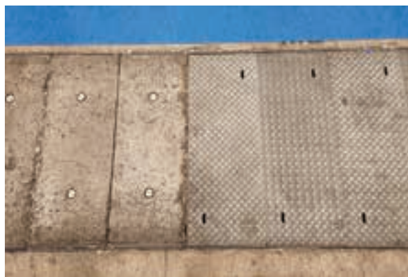
Electrical/Mechanical pit lids
